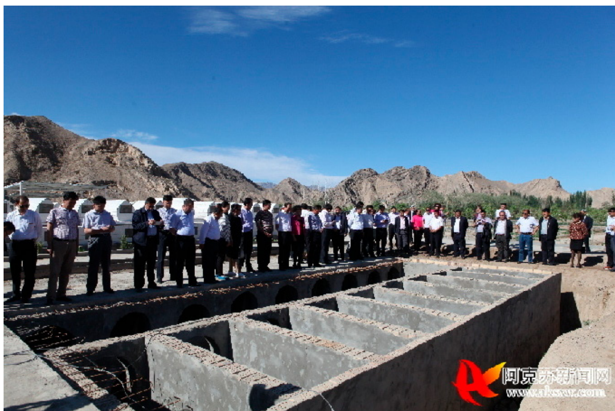
Figure 29: Mardan Mugai, Deputy Secretary of Aksu Prefecture’s Party Committee, and other members of the local government standing beside a ‘public welfare ecological cemetery’ construction site
