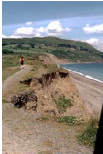
Plate 7 - Coastal erosion south of Bray Head - Co. Wicklow
