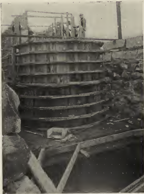
FIG. 21.—CONSTRUCTION VIEW OF THE WHEEL PIT. Showing the flume deck and the centering for the wheel pit.
