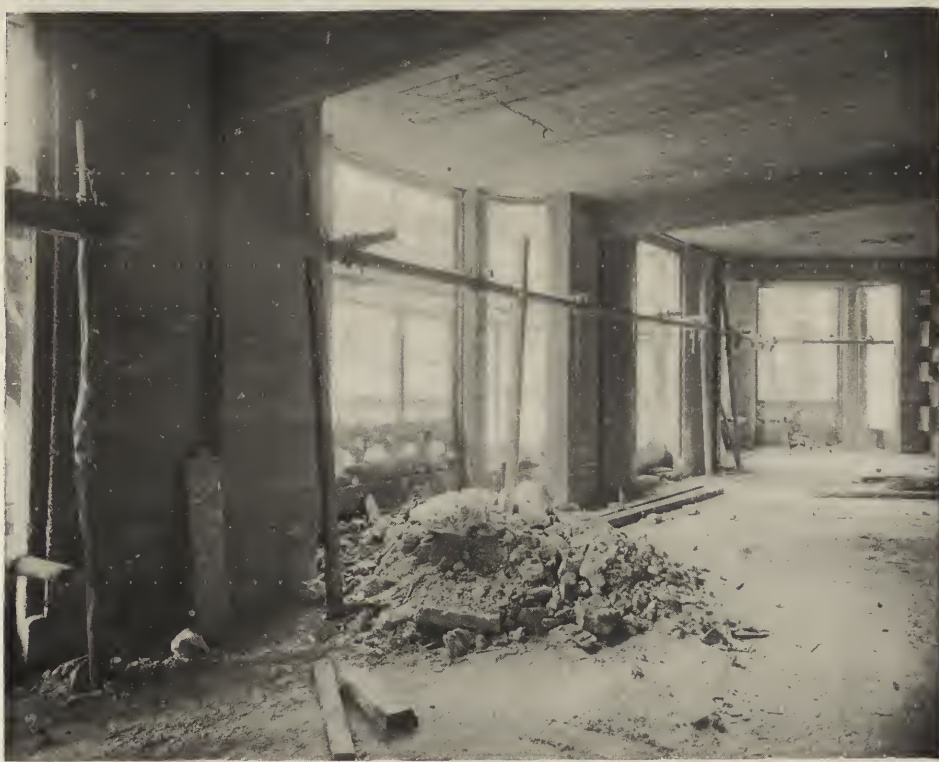
FIGS. 5 AND 6. THESE REPRODUCTIONS ALSO SHOW THE BUILDING AT NO. 1 RUE DAN- TON IN THE COURSE OF CONSTRUCTION. THE UPPER ONE REVEALS THE FLOOR CONSTRUCTION BETWEEN TWO STORIES, AND THE LOWER ONE THE ROOMS OF AN APARTMENT.
