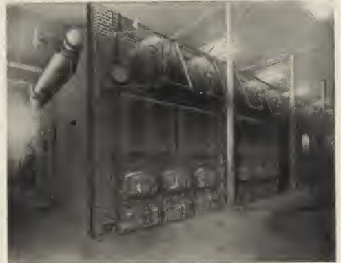
FIG. 39.—INTERIOR OF THE BOILER ROOM. Situated at the Elizabethport works of C. R. R. of N. J.
