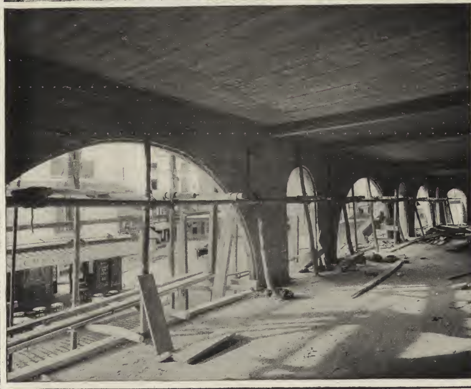
FIGS. 3 AND 4. THESE SHOW THE APARTMENT HOUSE AT NO. 1 RUE DANTON IN COURSE OF CONSTRUCTION. FIG. 3 ILLUSTRATES A MODEL FOR THE MOULD OF THE CORNICE ON THE SIXTH STORY. FIG. 4 SHOWS THE LARGE BAYS OF THE ENTRESOL.
