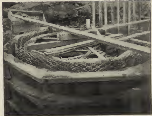
FIG. 19.—CONSTRUCTION OF A WHEEL PIT. This pit was situated at Walpole, Mass., and was 15 feet in diameter.
