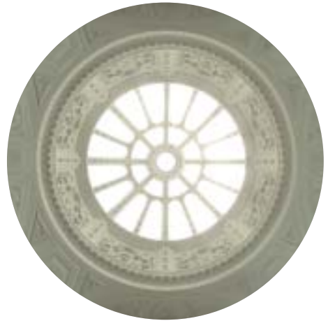
The 'dome' above the main staircase in the Old War Office Building seen from below
