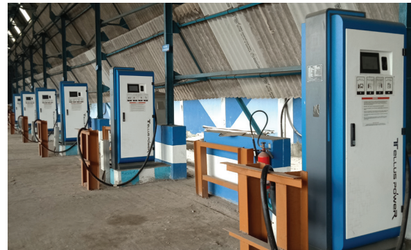
Figure 3: DC slow & fast chargers installed at Kasba bus depot in Kolkata
