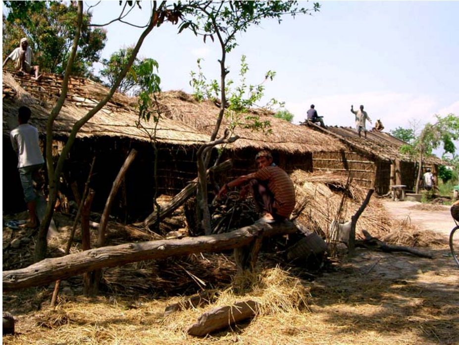
Plate 4.10 Gaas is still the main material for making roofs. Every year, people will repair their roofs before the monsoon season.
