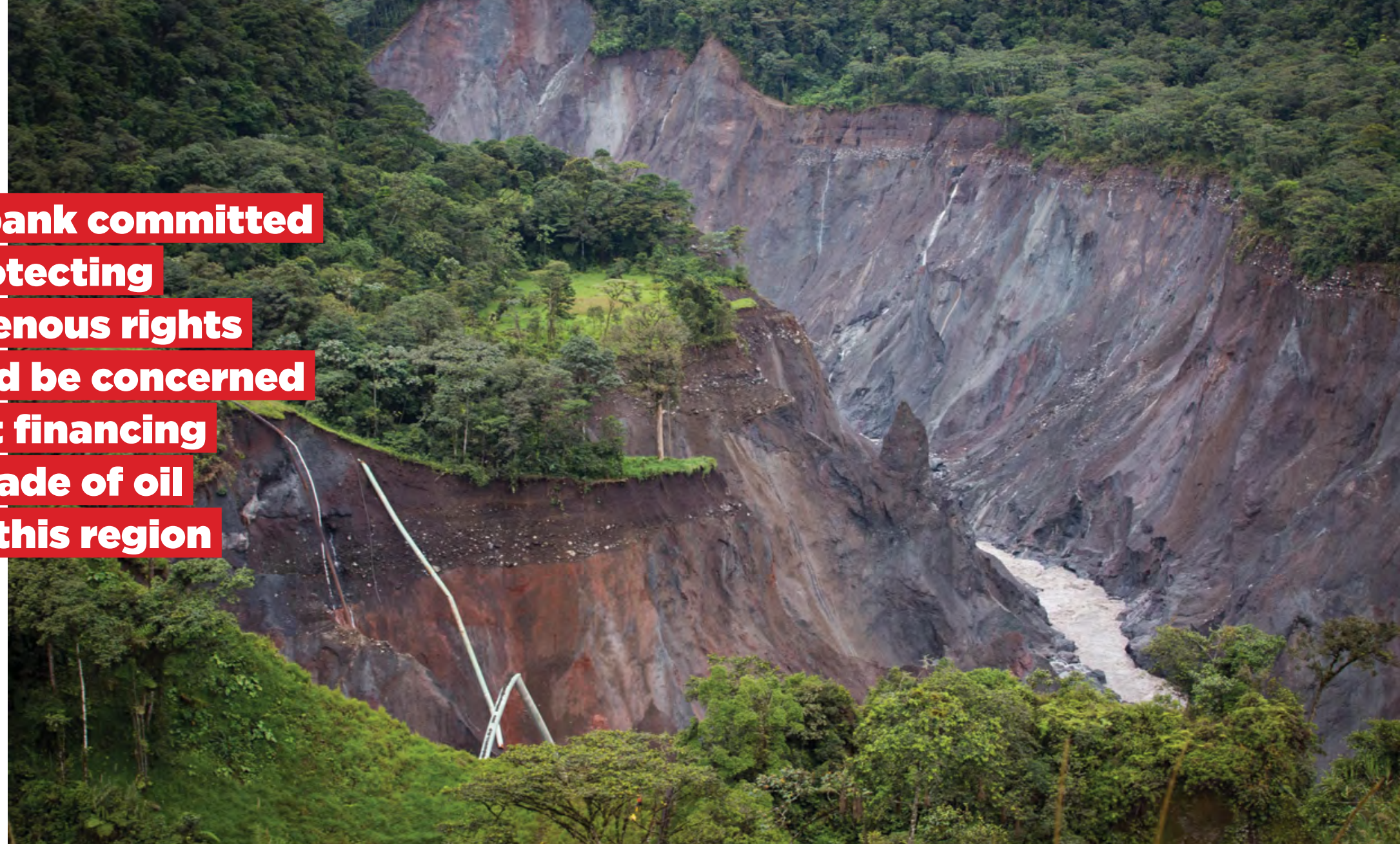
Repair work on the ruptured oil pipelines alongside the Quito-Lago Agrio road, Ecuador. IVAN CASTANEIRA/AGENCIA TEGANTAI
