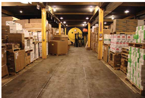
Figure 4.48. Example of unsuitable warehouse at McMurdo Station. In this warehouse, the forklift cannot be driven in some areas because breakthroughs and other floor damage have occurred. Source: USAP photo archives.
