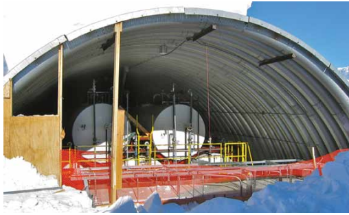
Figure 2.6. The fuel storage facility at South Pole Station. Source: Carlton Walker.
